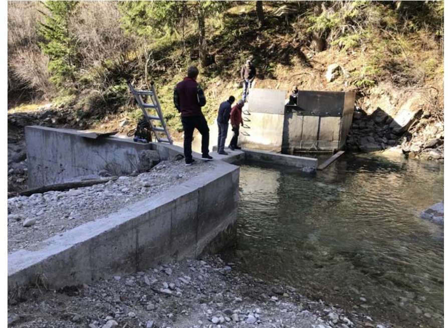
New plating at the Glenwood Springs water intake on Grizzly Creek was installed by the city to protect the system's valve controls and screen before next spring's snowmelt scours the Grizzly Creek burn zone and potentially clogs the creek with debris. (Provided by the City of Glenwood Springs via ColoradoSun.com)
